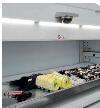
External bay lighting
